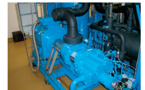
Ethylene Glycol chiller unit
